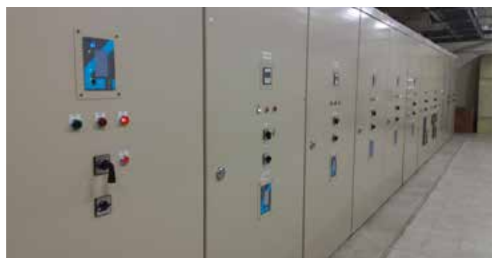
AQ F215 feeder protection IEDs installed in 23.9kV panels.
